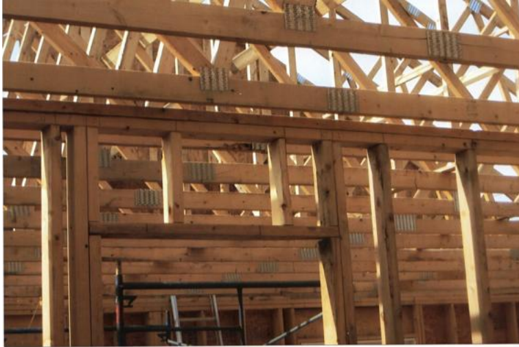
Unsupported interior partitions. Furring strips should be added before interior partitions are attached.
