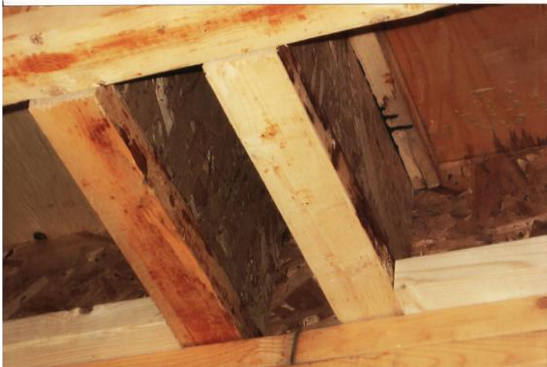
Rim joist missing and improper framing
