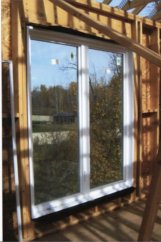
Bottom of window very low, a concern for person falling out the second floor
